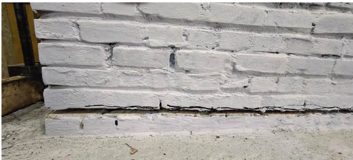
Figure 4.2- Cracks at final state of SURM4 (Sliding).
