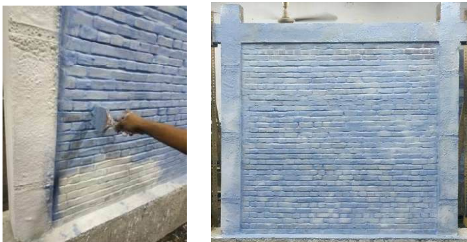
Figure 3.29- Infilled Frame after whitewash.
